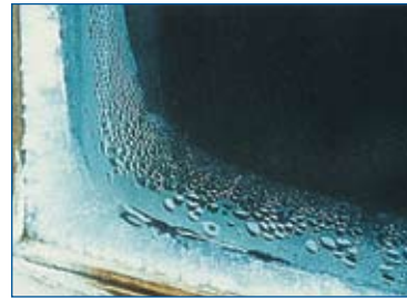
Window condensation can fuel mold growth.
